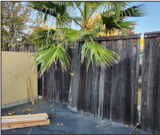
The old fence. The contractors (Aguilar Fence, Inc.) were able to demolish the old fence, remove a palm tree that had overgrown into the fence (with the help of a subcontractor), cut away old posts, install new steel posts into fresh concrete, and build the new fence all in a single day!
